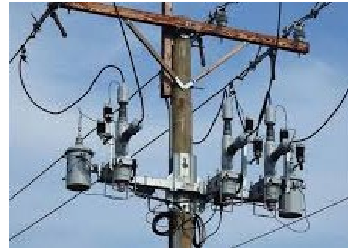
Automated Recloser Switch Source: T&D World
