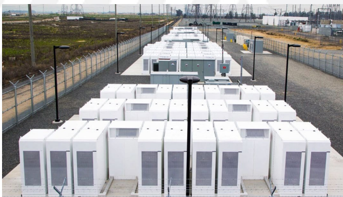
SCE's 20 MW, 4-hour storage plant in Mira Loma, CA
