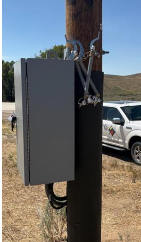
Fire protective wrap
