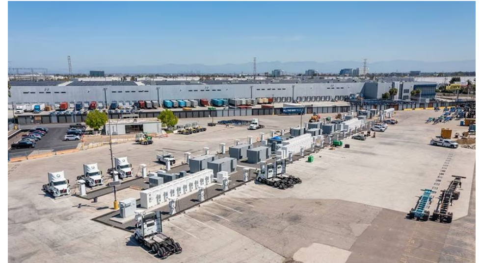
A 9 MW microgrid charging solution near the Port of Los Angeles. Capable of charging 96 EV trucks simultaneously. Owned by Prologis to serve Maersk's drayage truck fleet.
