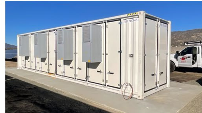
Resiliency-scale storage (5MW/20MWh)
