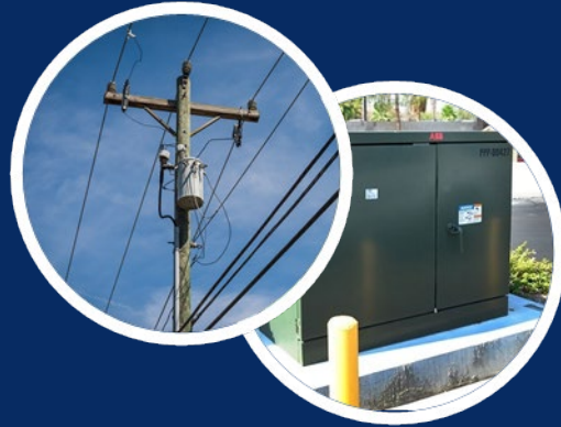
Service line and transformers
