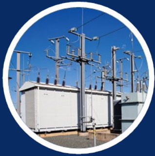
Upstream distribution network and substations
