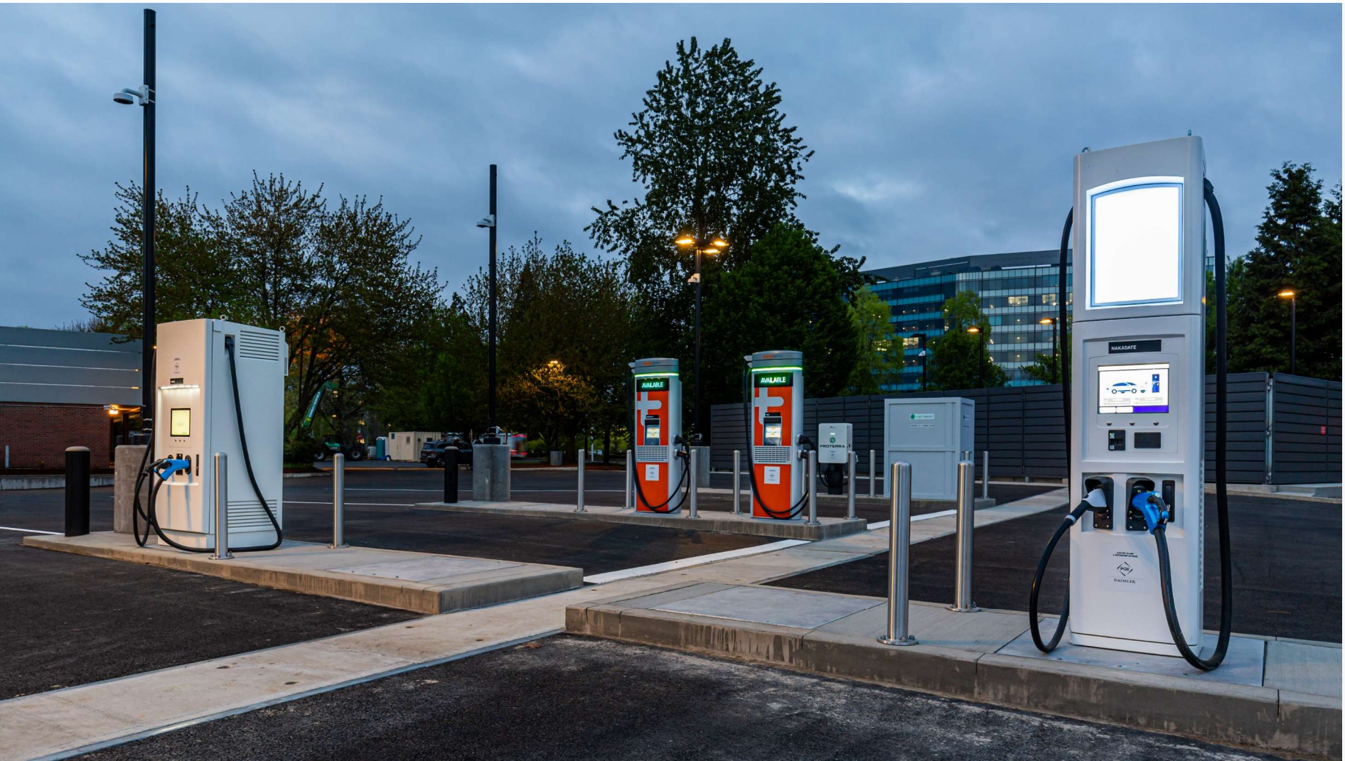
Finished site - note the extra bollards to prevent any accidents during truck maneuvering
