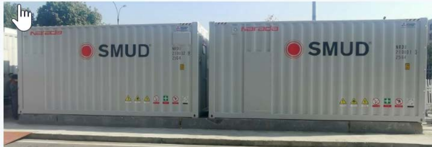
Two of the 6 energy storage units destined for our Hedge site in south Sacramento County.
