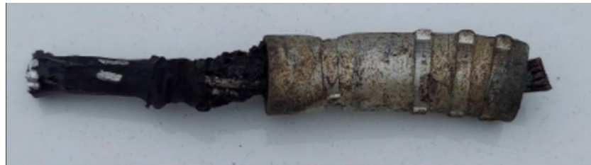
Example of a bad (but not yet failed) electric grid component found during pilot
