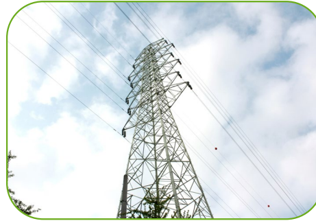
Safety/Risk for Traveling Public
