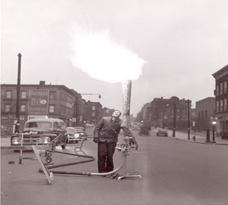
A purge burner igniting manufactured gas being replaced in a main by natural gas during the 'great conversion' in 1952
