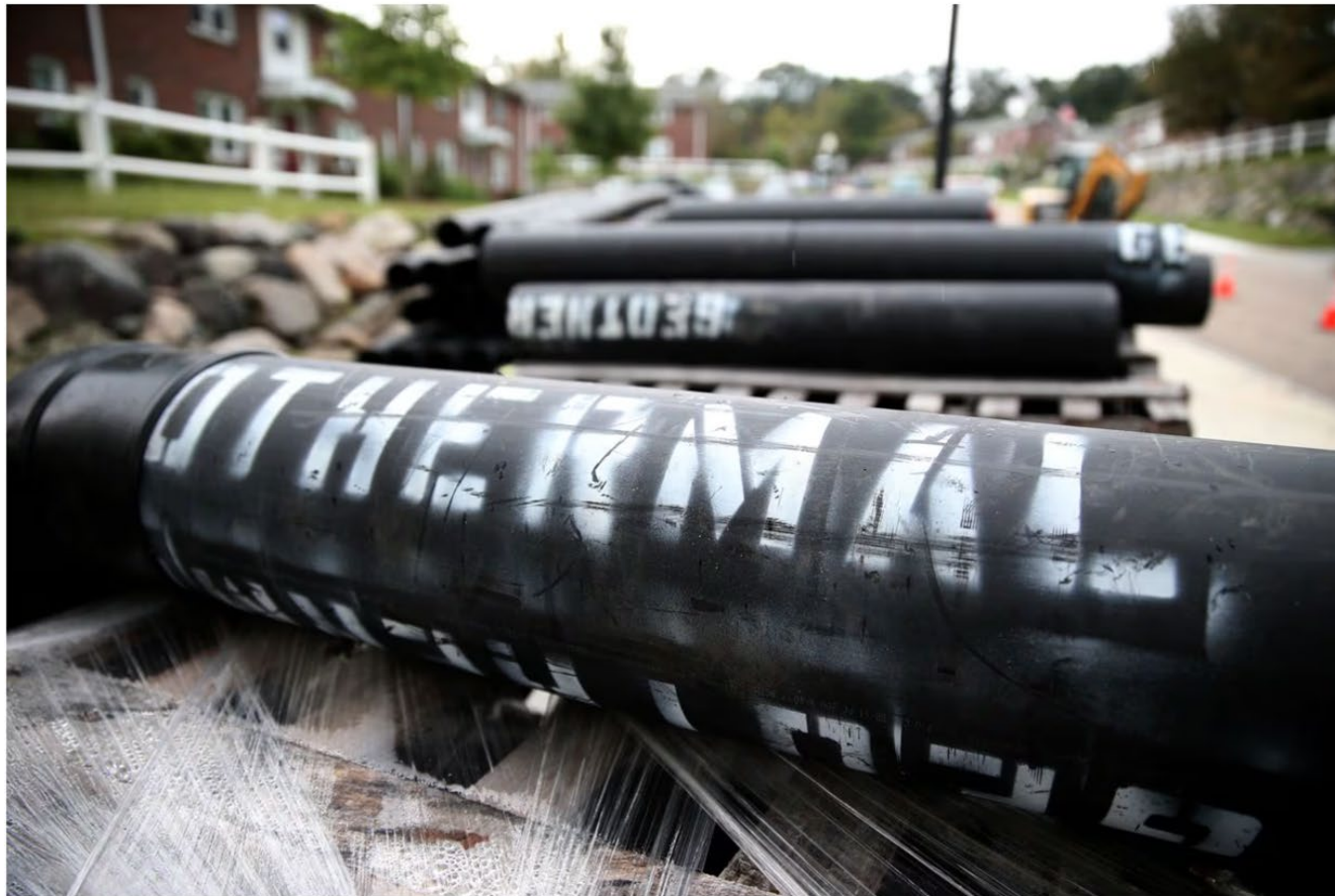
Geothermal pipes were ready for installation in 2023 for Eversource's geothermal networking pilot program in Framingham. JONATHAN WIGGS/GLOBE STAFF
