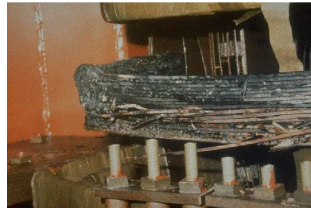
GSU Transformer from Salem
